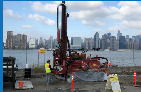
ADT provides geotechnical and environmental drilling services to the greater New York City area.
